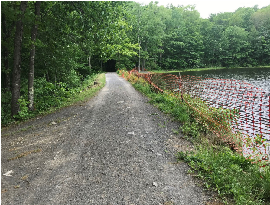
Figure 3-2 View along carriage road on crest of dam, looking south (photo by SLR)
