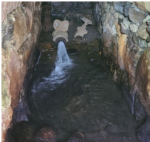
Figure 3-11 Inoperable low-level outlet valves (photo from Mohonk files)
