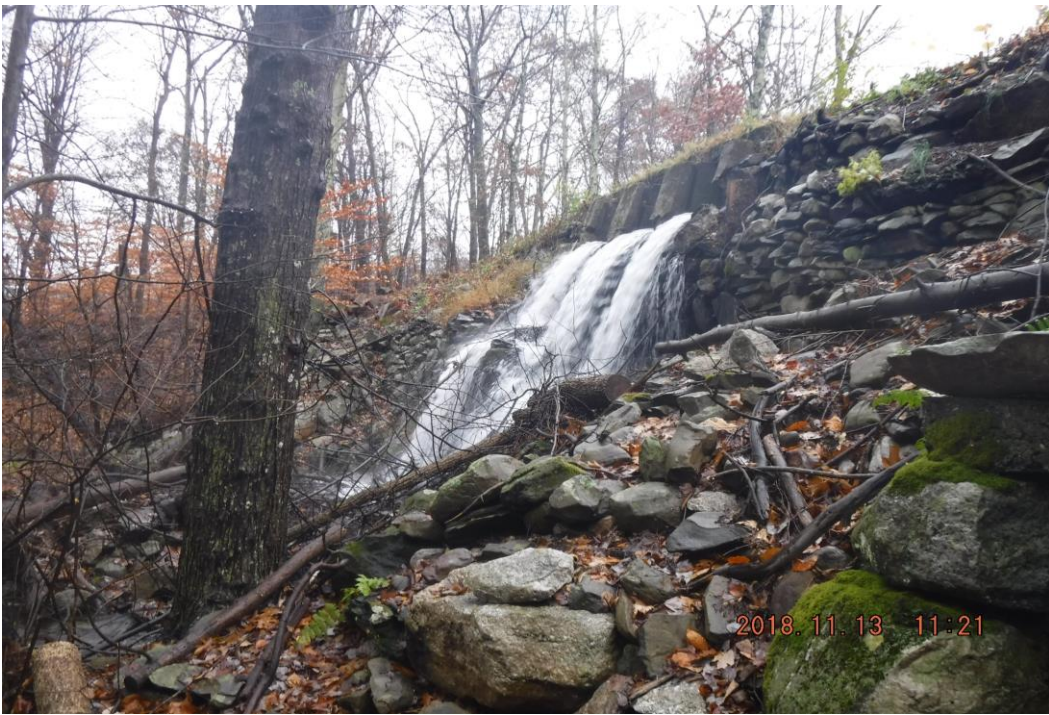
Photo 8 Dam ID# 193-5962 Duck Pond Dam 11/13/2018 Downstream spillway face View looking right from downstream toe
