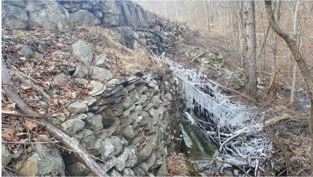
Figure 3-3 View of downstream face of dam, looking north (photo provided by Chuck Reid)
