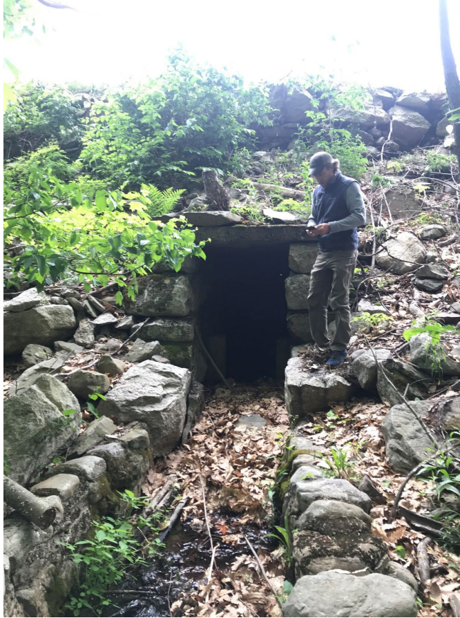
Figure 3-10 Low-level outlet chamber in downstream face of main dam (photo by SLR)
