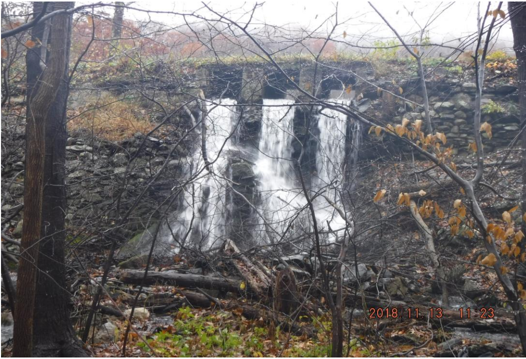
Photo 7 Dam ID# 193-5962 Duck Pond Dam 11/13/2018 Service spillway downstream face View looking upstream
