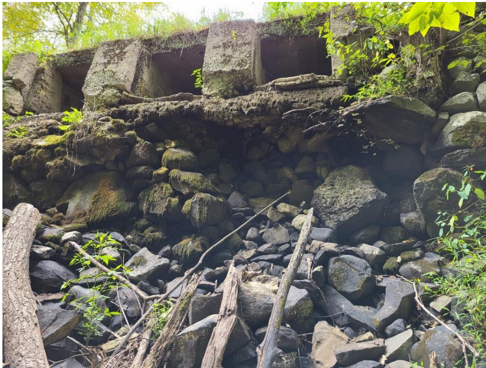
Photo 2 Missing masonry, large void, and undermined spillway section (looking upstream at downstream face)
