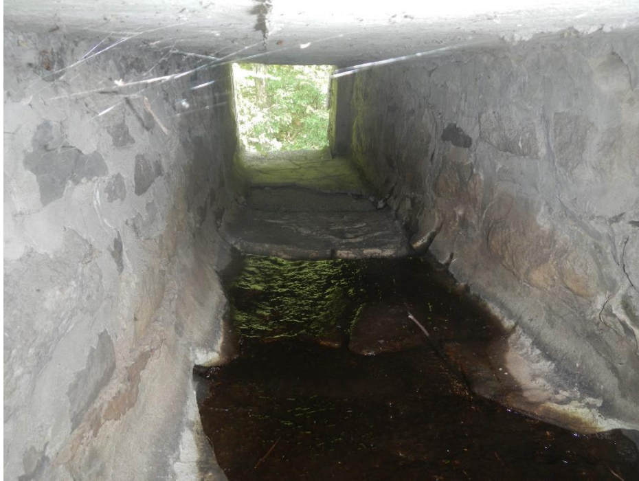
Photo 1 Spilling flows entering lateral crack in base of spillway section (looking downstream through right spillway section)
