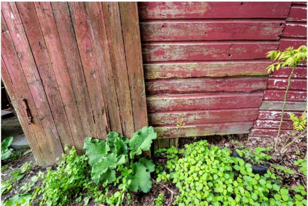
#B2-6 Brook Farm Barn 2 North Lower Level, 60 Gatehouse Road, New Paltz, NY 12561, 5/8/2024, Ulster
