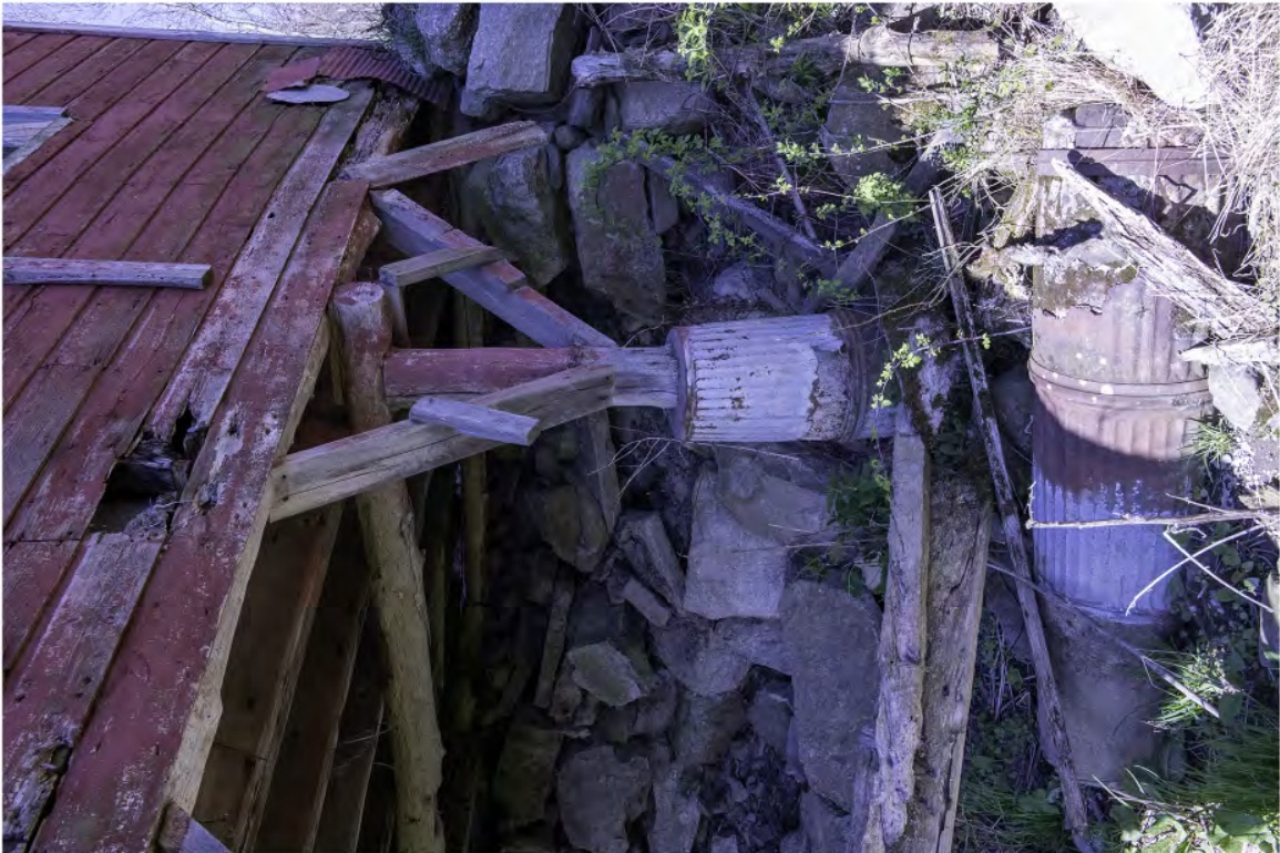
#B3-5 Brook Farm Barn 3 Northwest underneath, 60 Gatehouse Road, New Paltz, NY 12561, 4/25/2024, Ulster
