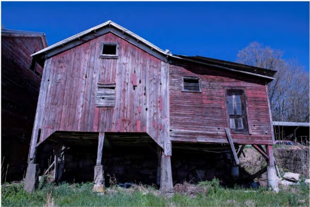
#B3-17 Brook Farm Barn 3 East Underneath, 60 Gatehouse Road, New Paltz, NY 12561, 4/25/2024, Ulster
