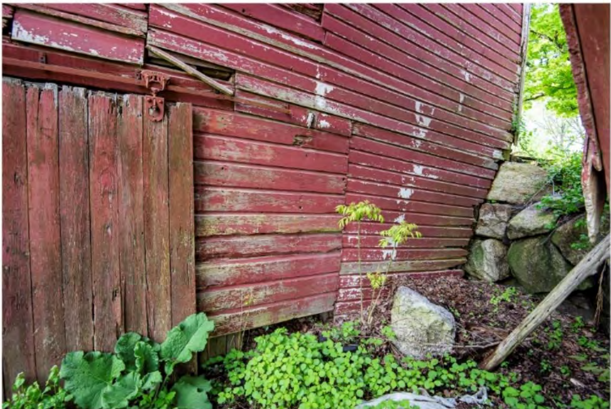
#B2-2 Brook Farm Barn 2 Northeast Lower Level, 60 Gatehouse Road, New Paltz, NY 12561, 5/8/2024, Ulster
