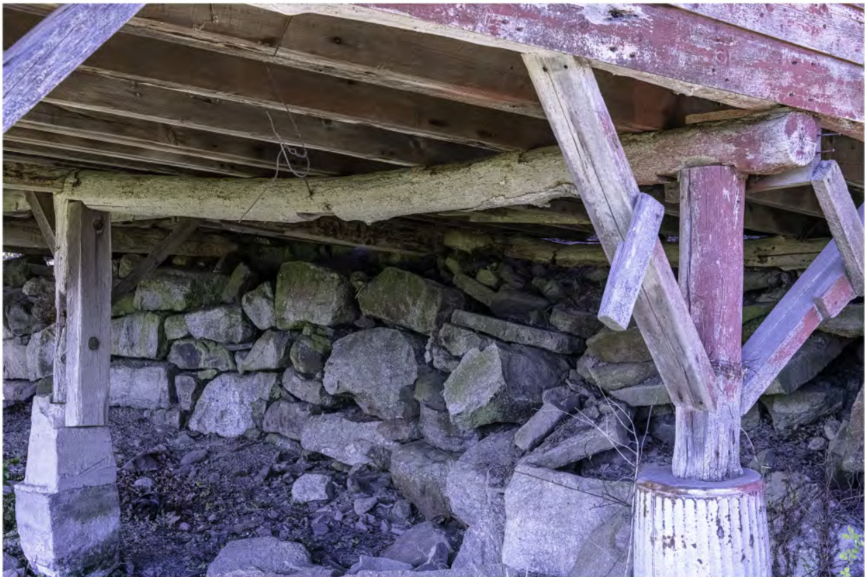
#B3-11 Brook Farm Barn 3 Northeast underneath, 60 Gatehouse Road, New Paltz, NY 12561, 4/25/2024, Ulster
