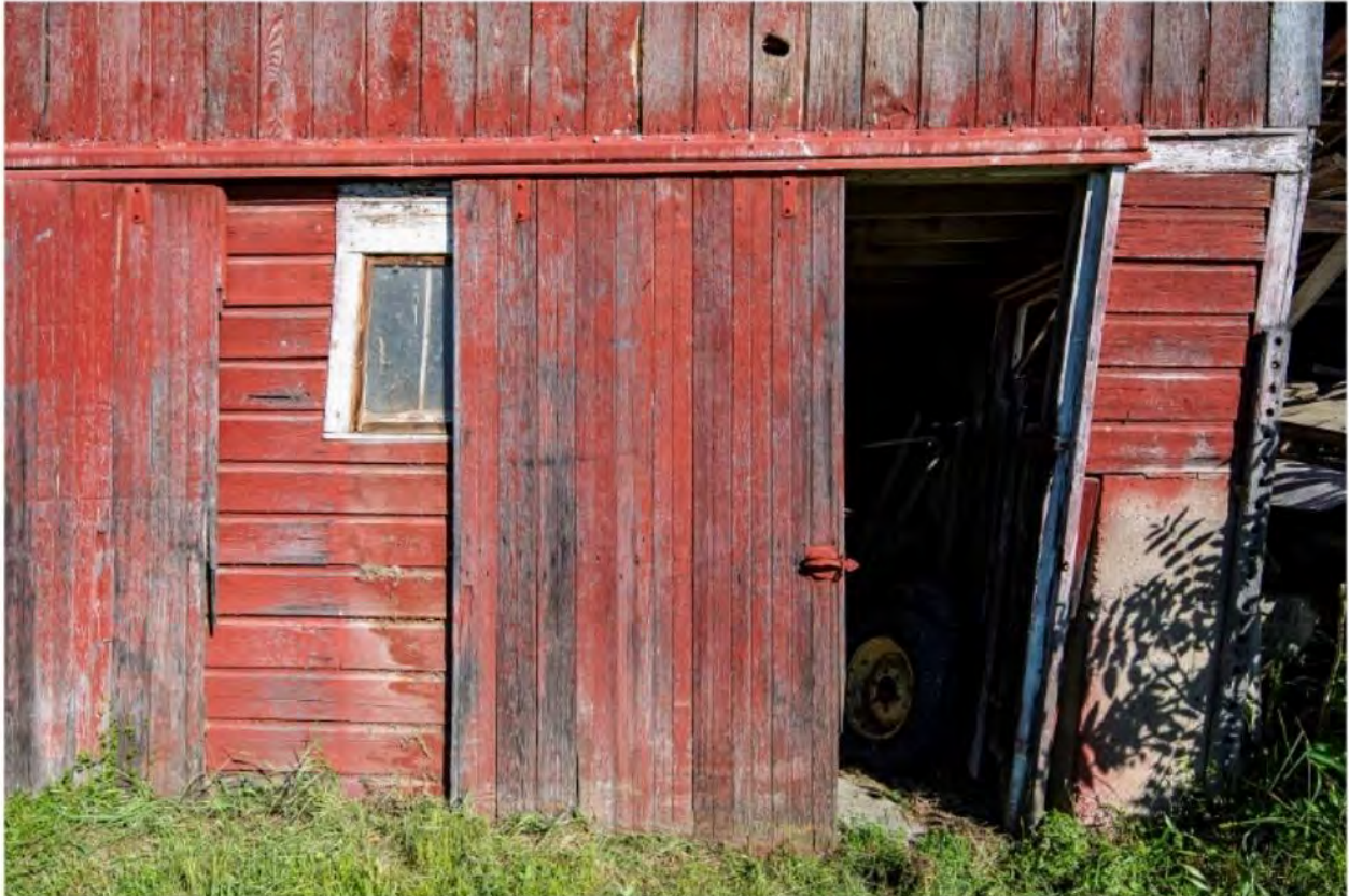
#B1-10 Brook Farm Barn 1 Northeast Door, 60 Gatehouse Road, New Paltz, NY 12561, 6/8/2024, Ulster
