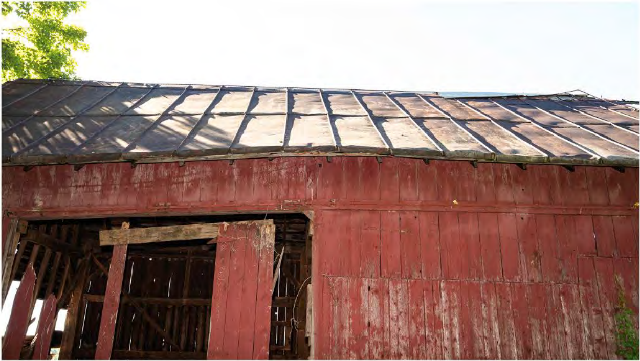
#B1-1 Brook Farm Barn 1 West Roof, 60 Gatehouse Road, New Paltz, NY 12561, 6/8/2024, Ulster
