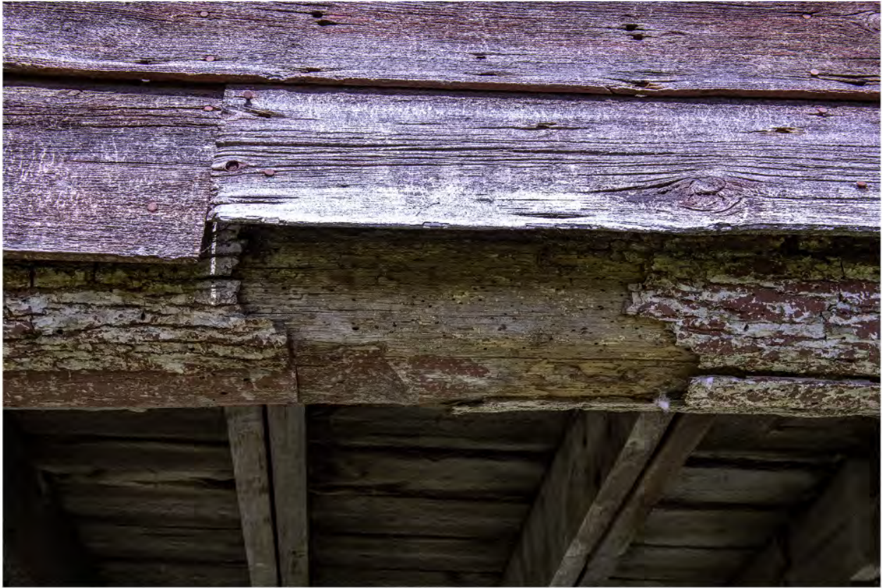
#B3-14 Brook Farm Barn 3 East Underneath, 60 Gatehouse Road, New Paltz, NY 12561, 4/25/2024, Ulster
