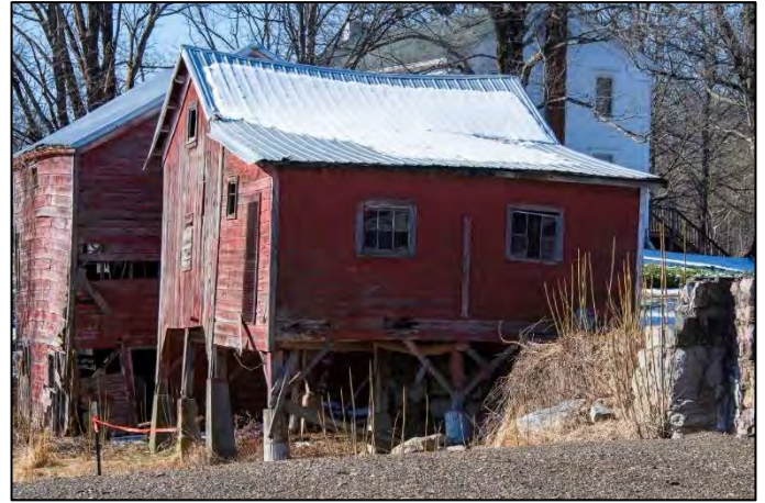
Fig. #85 Brook Farm Barn 3 Weathered Siding
