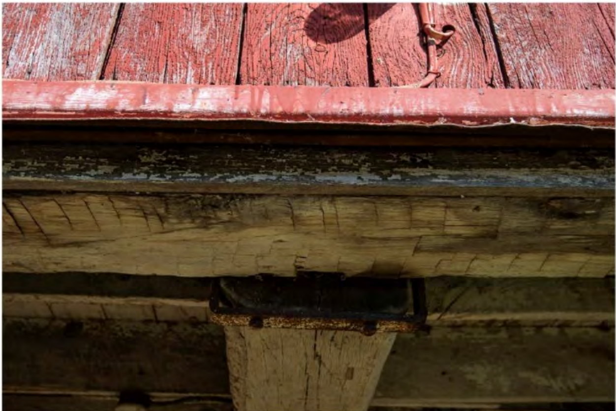
#B1-74 Brook Farm Barn I hardware, 60 Gatehouse Road, New Paltz, NY 12561, 6/8/2024, Ulster
