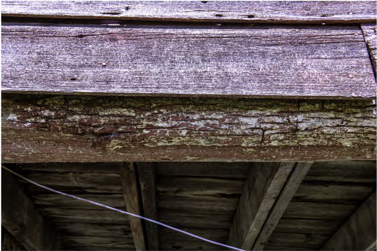
#B3-13 Brook Farm Barn 3 East Underneath, 60 Gatehouse Road, New Paltz, NY 12561, 4/25/2024, Ulster
