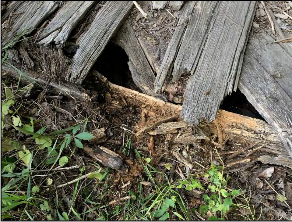
Photo 25-Barn 4: View of heavily deteriorated sill plate at Barn 4.
