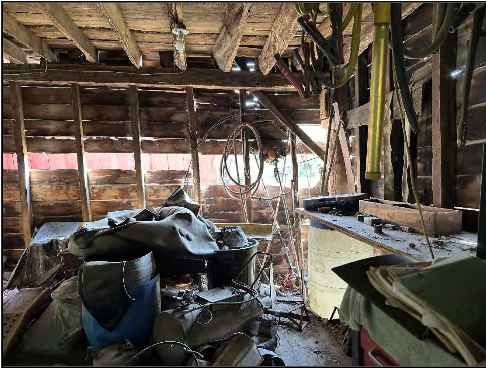
Photo 13-Barn 2: View of wall with missing sheathing. This has allowed the building to be subject to rain, snow, and sun exposure.
