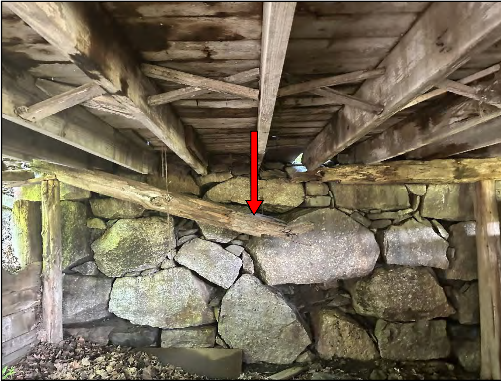
Photo 15-Barn 2: View of stone retaining wall with no mortar and visible gaps. View of edge support beam that has dynamically failed.
