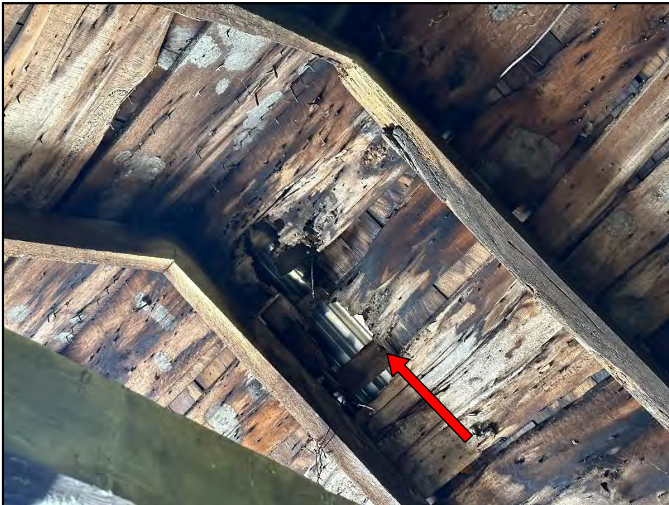
Photo 10-Barn 2: View of undersized rafters with no ridge board in Barn 2. Significant deflection is present and some rafters show signs of section loss. Also view of highly deteriorated roof sheathing that has been covered with corrugated metal roofing. This condition is typical throughout.
