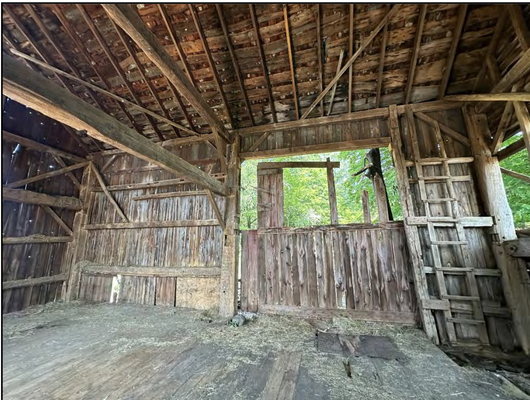
Photo 4-Barn 1: View of Western wall with non-functioning door. All walls at this level contain little-to-no lateral bracing.
