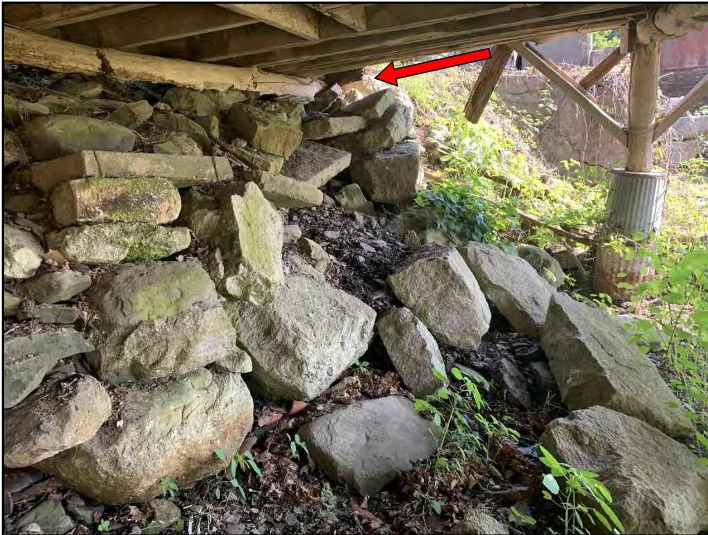
Photo 20-Barn 3: View of stone retaining wall at Barn 3. The wall has failed and caused significant settlement to the building.
