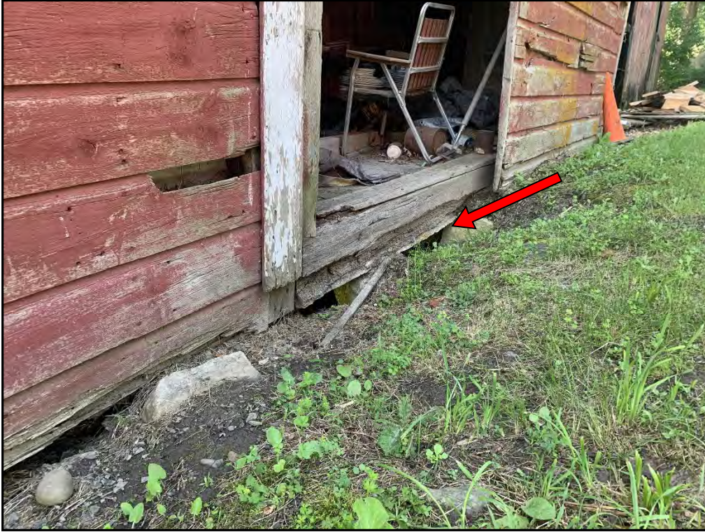
Photo 19-Barn 3: View of erosion at the deteriorated sill of Barn 3. This is creating a gap between the stone retaining wall and the wall of the barn.
