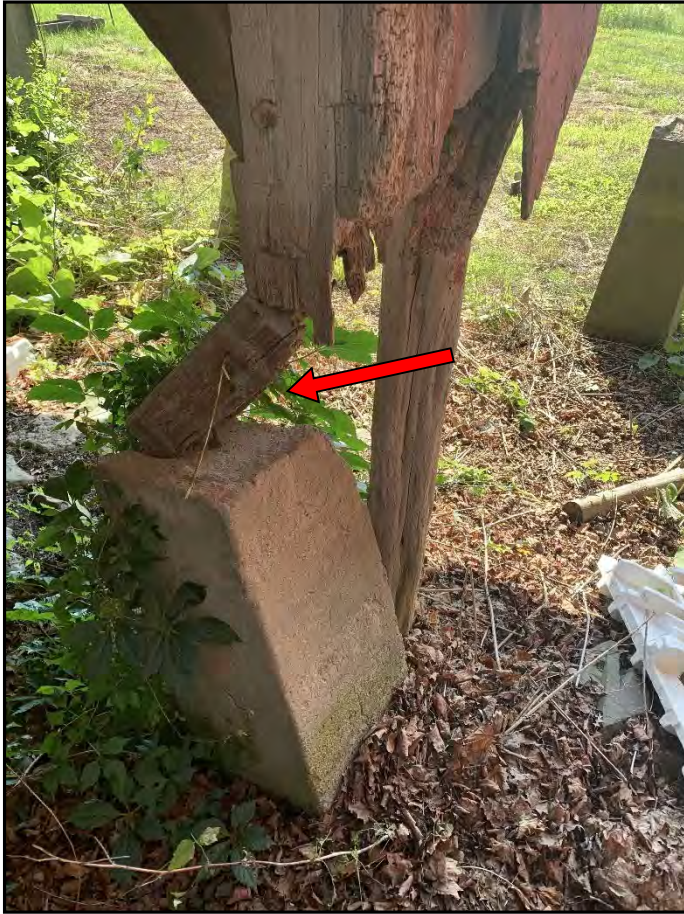
Photo 21-Barn 3: View of failing concrete pier. Framing above this location is essentially unsupported.
