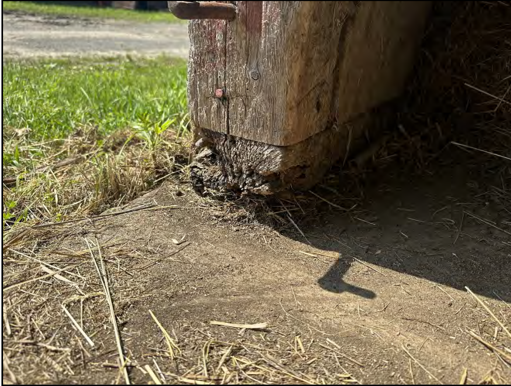
Photo 7-Barn 1: View of deteriorated sill plate in Barn 1. This has caused significant settlement to the building.
