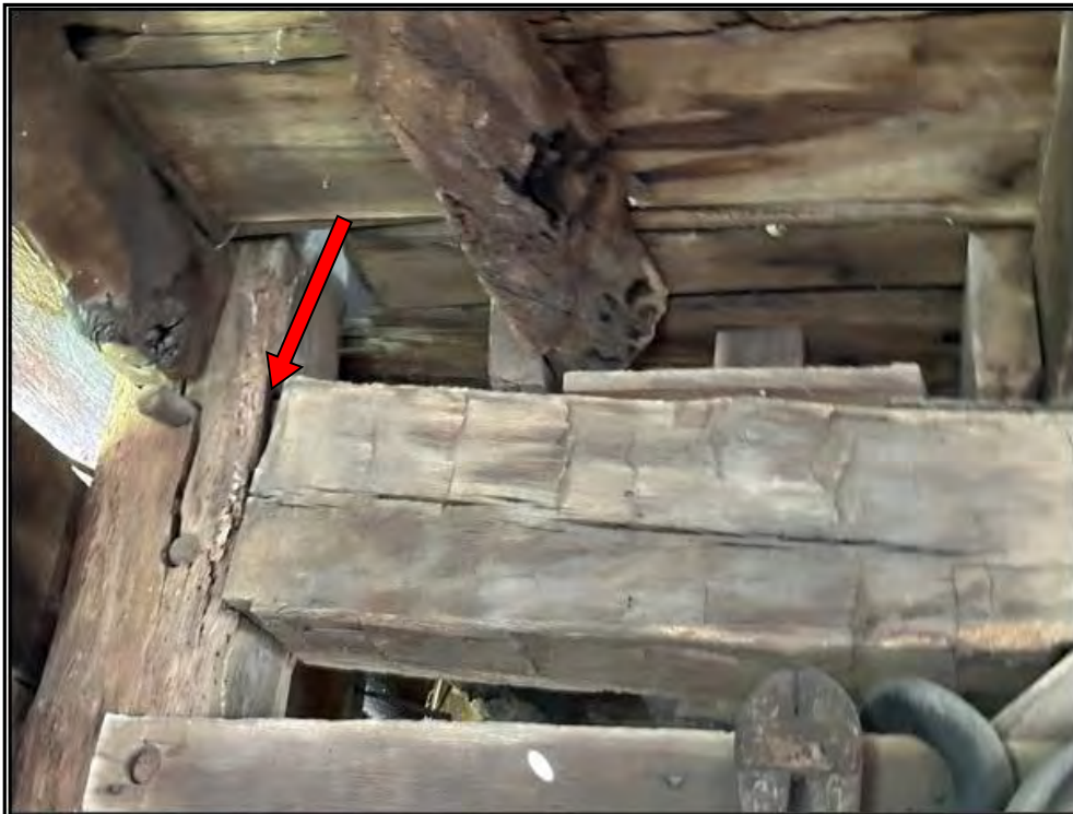
Photo 12-Barn 2: View of failing main support beam connection.
