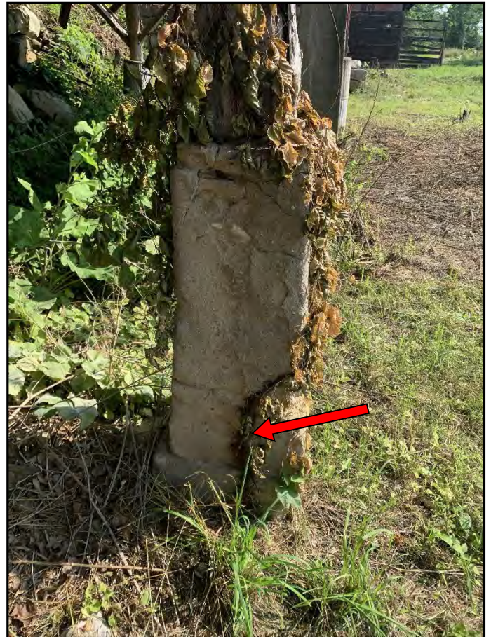
Photo 22-Barn 3: View of cracked concrete pier.
