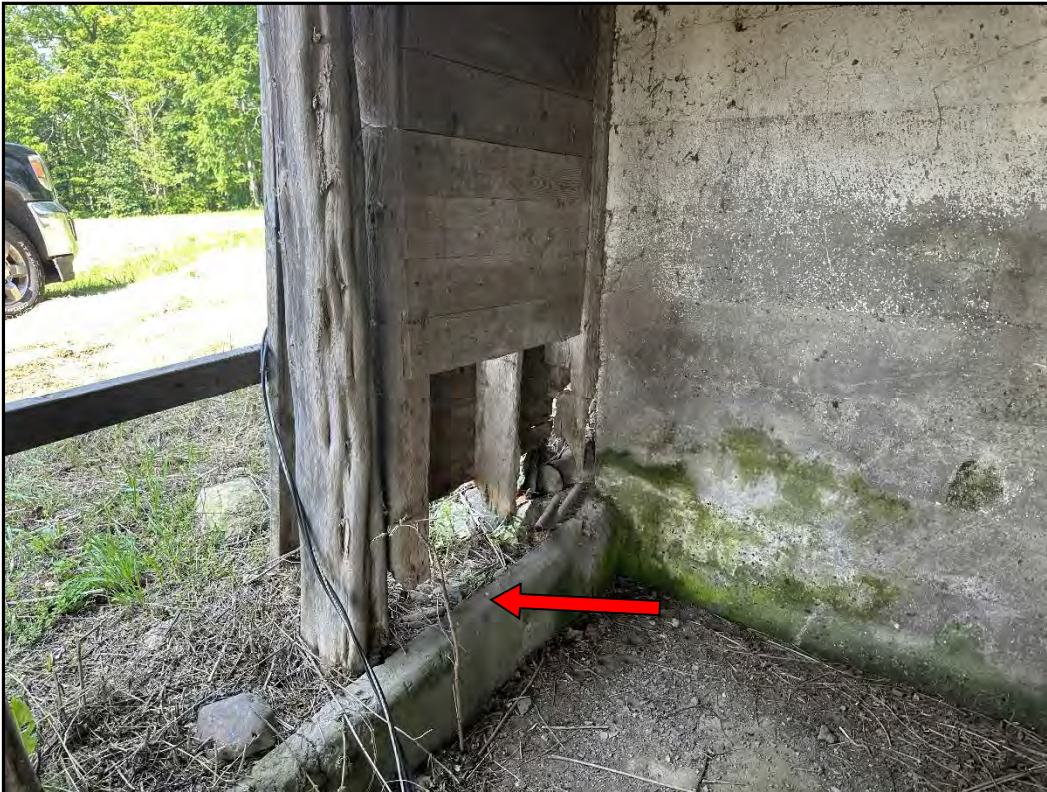
Photo 8 Barn 1: View of wall studs significantly deteriorated an no longer in contact with the sill plate or the ground.
