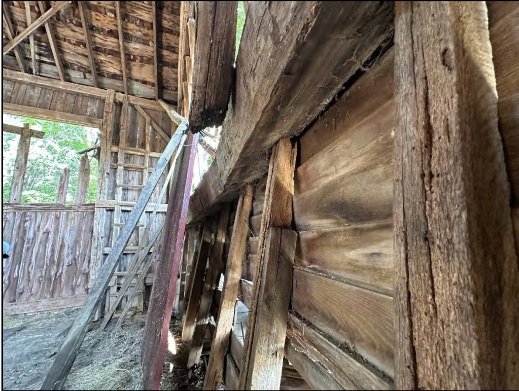
Photo 5-Barn 1: View of significant movement and deterioration in the Northern bent.
