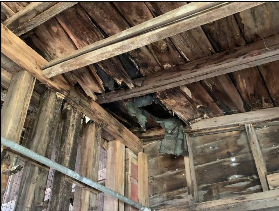
Photo 18-Barn 3: View of highly deteriorated roof sheathing.
