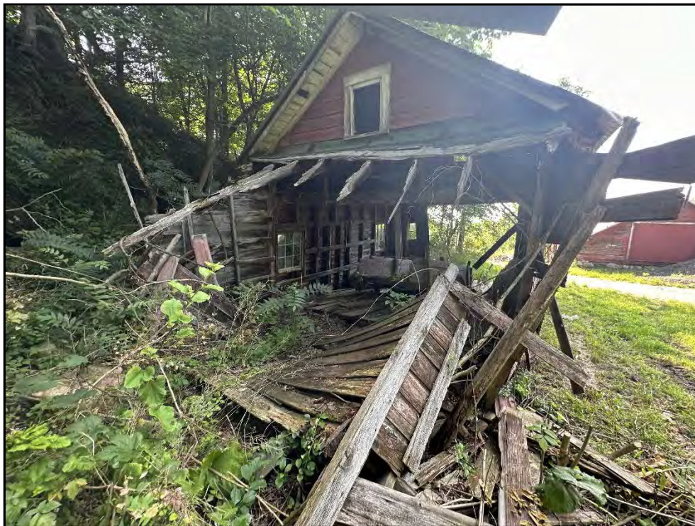
Photo 24-Barn 4: View of collapsed portion on rear side of Barn 4.
